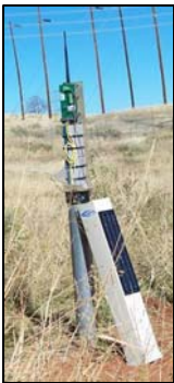
FGRCP Line Marker Test Station
