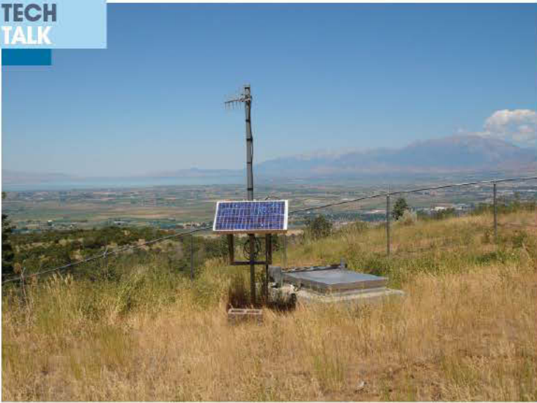
Carefully selected locations for remote terminal units are important to the design of a wireless SCADA system.
