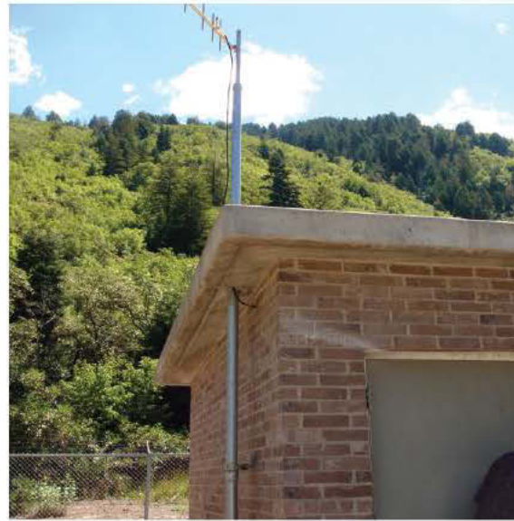
Wireless SCADA enables control of widely scattered field sites without the costs and limitations of hardwired systems.
